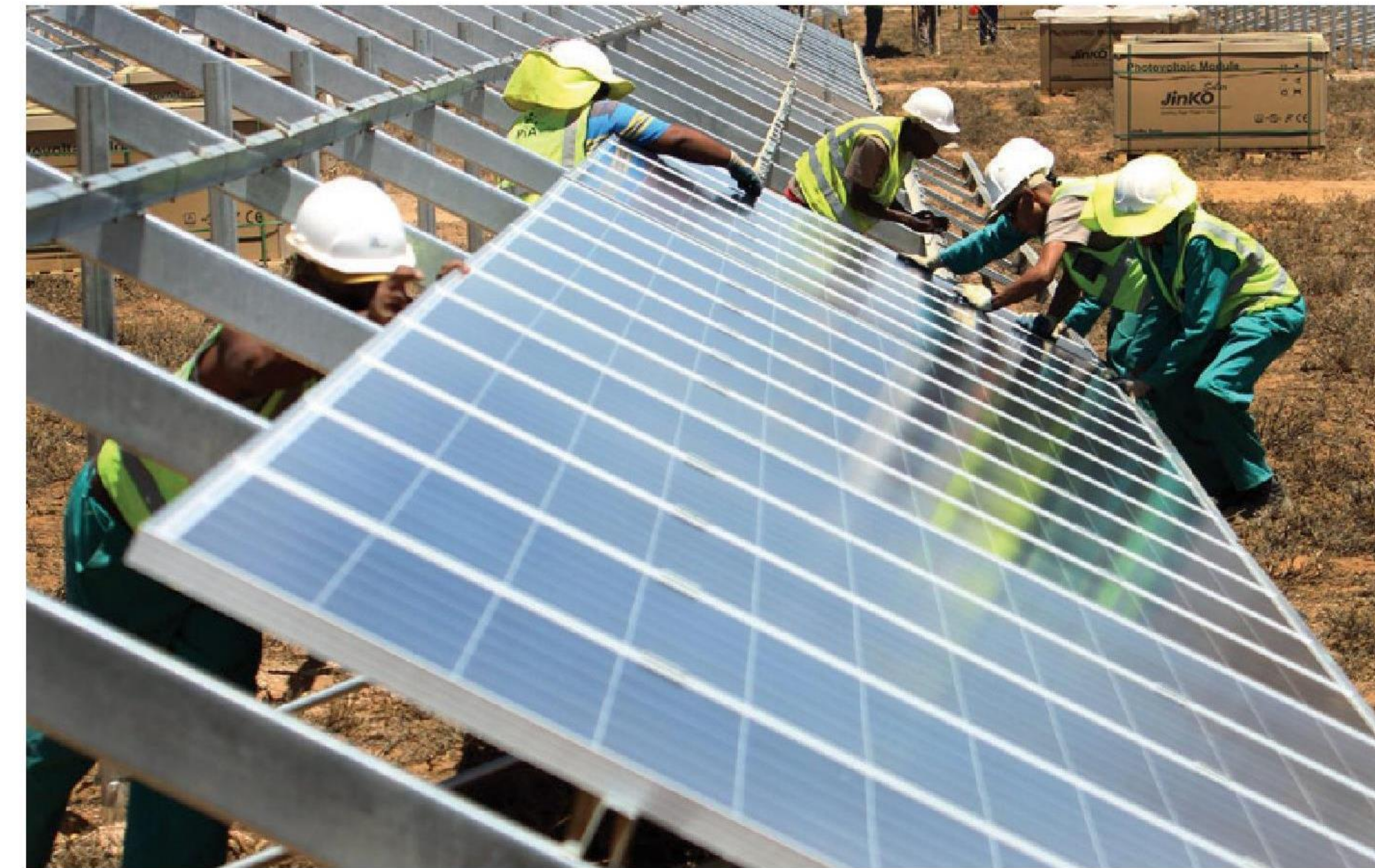
CHANGE TO SOLAR ENERGY: Workers fit a solar panel in De Aar, Northern Cape.
